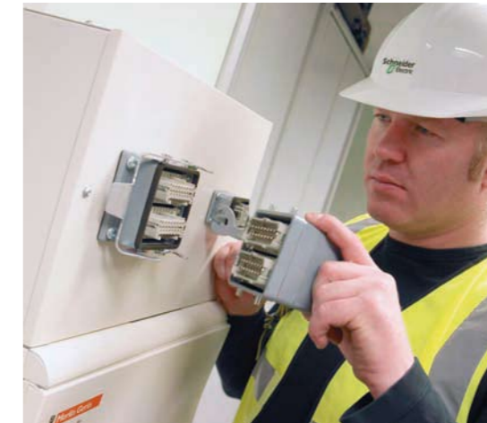
Dramatically reduce installation times with our reliable 'plug and play' technology – pre-built and pre-tested by Schneider Electric.
